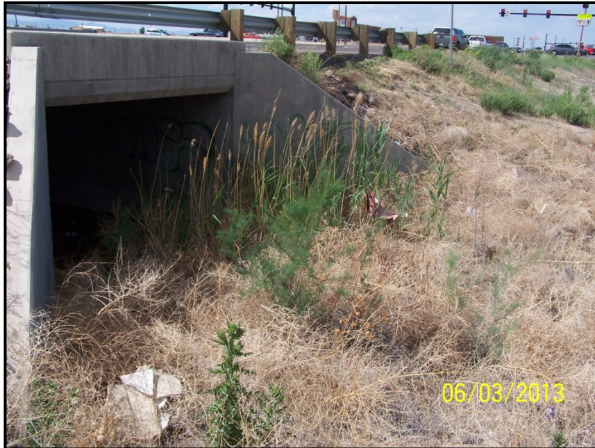
Photo 11 — Looking north next to the concrete box culvert under Purcell Blvd, for the tributary to Williams Creek. This drainage is highly channelized and filled with noxious weeds.
